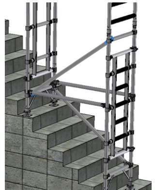
6) Fit another diagonal from the bottom rung of the plain portal frame to the top rung of ladder portal frame on the right hand side.
